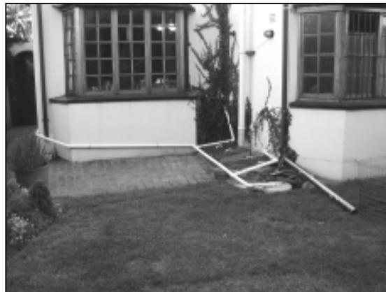
Pipes for greywater recycling are led to a sump, the water being used to spray the garden
